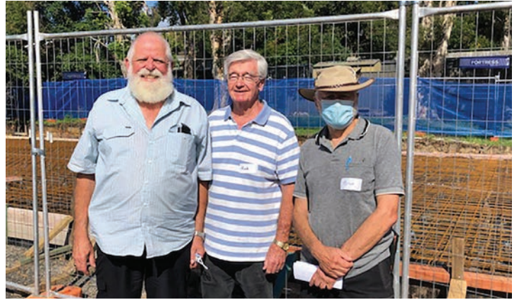
Above: Pictured at the Shed construction site after the AGM are NEMS President Brian Bailey, Community Bank Epping Chairman Rob Phillips, and NEMS Committee Member Peter Youll. Above left: Artist impression of finished building. Below: Progress is being made at the construction site.
