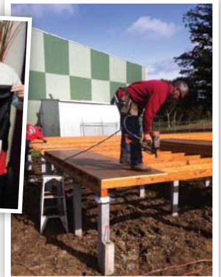
▲ Above: Construction taking place on the new clubrooms. Above left: Director Graham Stewart and Branch Manager Jason Chuck presenting Riddell's Creek Football Club with their grant.
